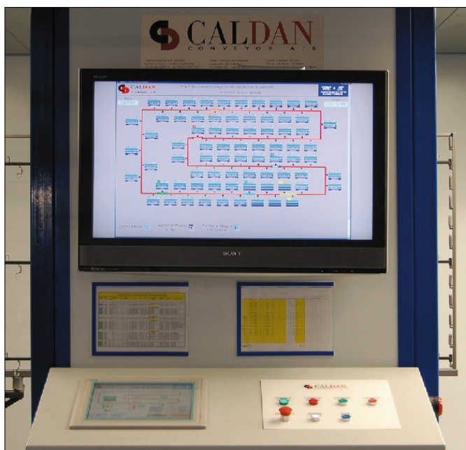
The paint plant is masterminded by a sophisticated process management system, which controls and monitors the finishing process throughout all its stages. The focal point of this "total interface" is a 42in plasma screen display and control panel in the load/unload zone.
