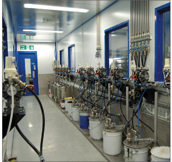
The paint mixing and distribution room. The ITW Binks equipment was supplied by Sedco (North West). Like most of the installation, this section utilised standard modular panels from Delta Process Systems.
